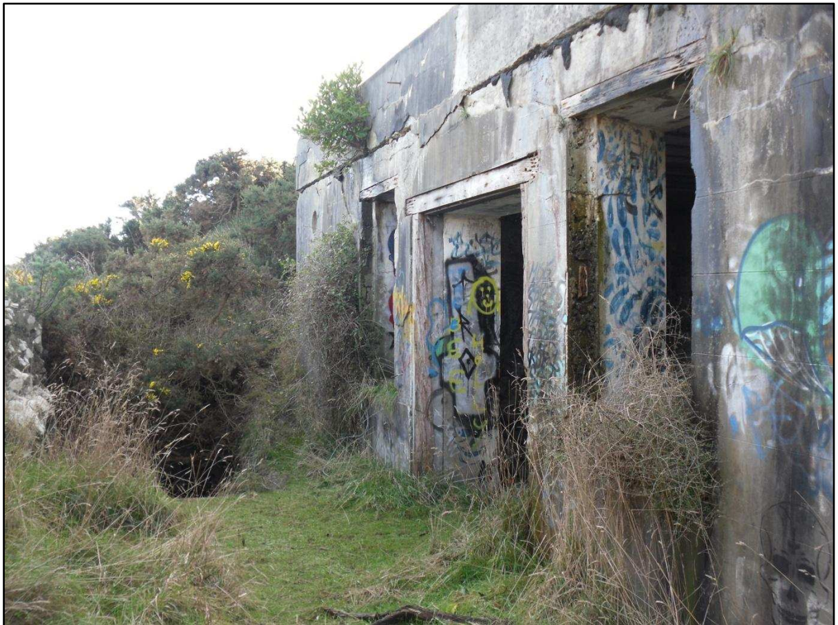
Figure 12. 1890s Engine Room. Facade has partially deteriorated, revealing concrete construction underneath.
