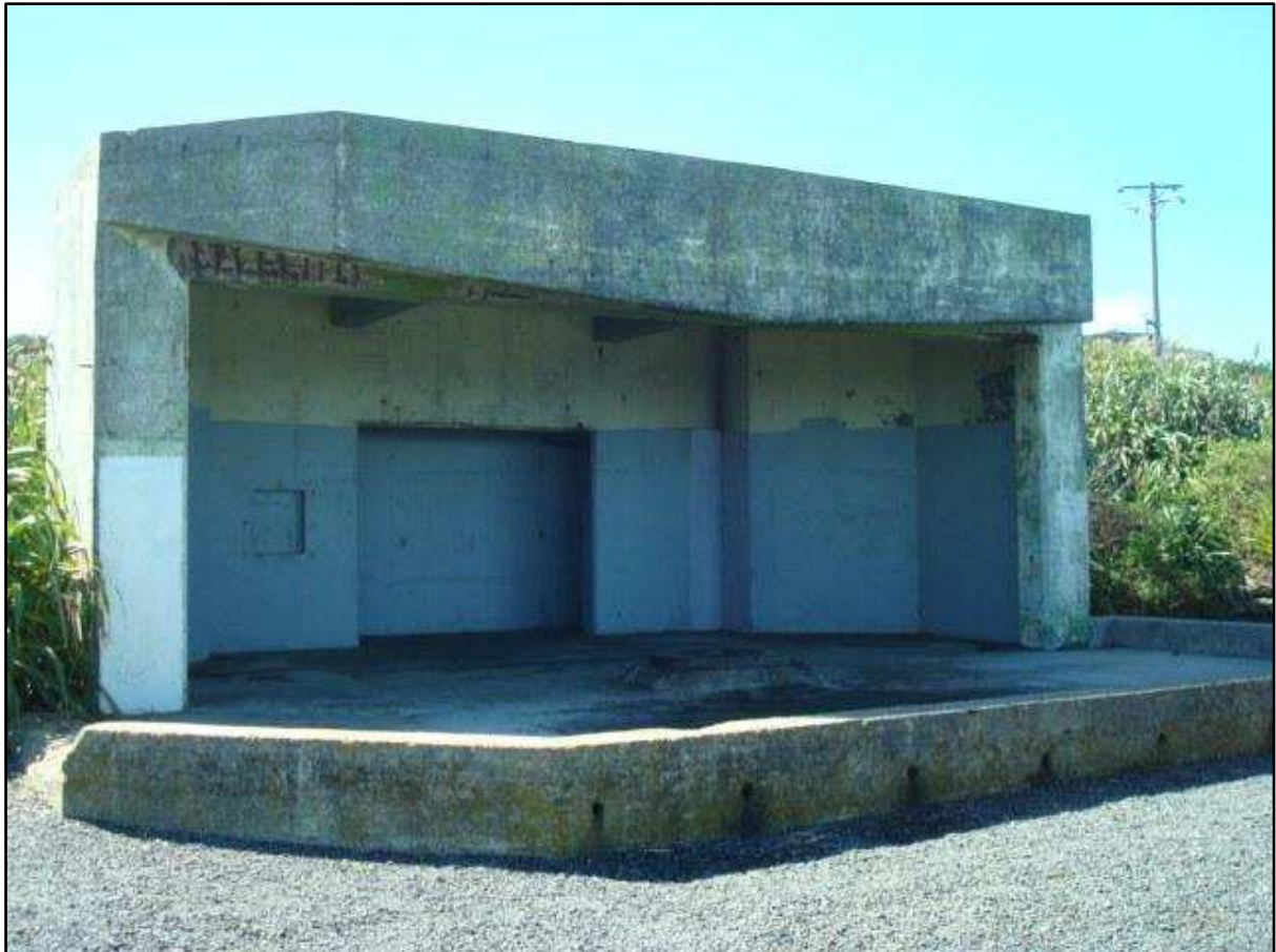
Figure 18. Tomahawk 6-inch Gun Emplacement. Minimal deterioration can be seen in upper left section of canopy with metal reinforcement revealed from within the concrete.
